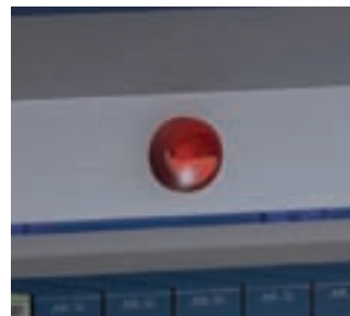
Operation indicator beacon.
